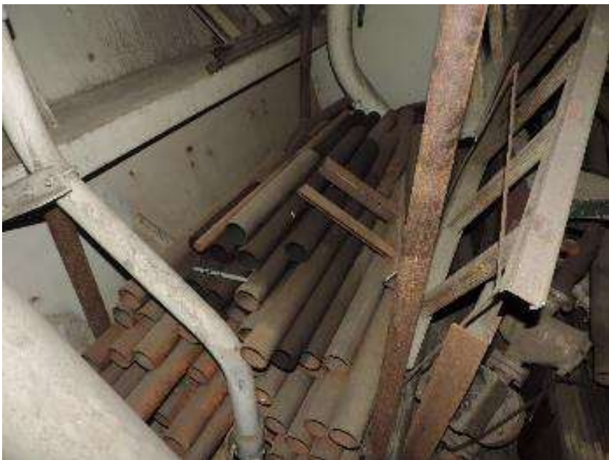
Figure 20.7 Steel pipes considered suspicious by KSA (Panel on 25 December 2017)
